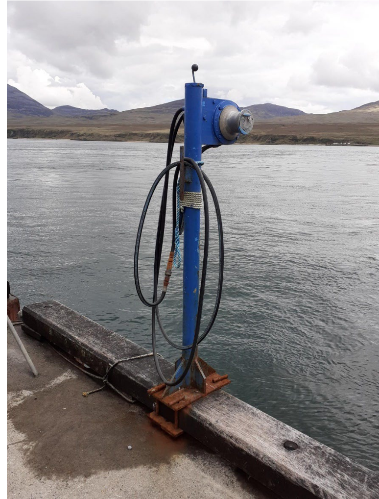
Image B8. Port Askaig, equipment inappropriately fixed
